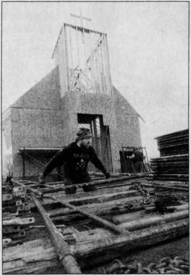
Greg Peer, center, and Roger Ostrenga, background, of Ostrenga Excavating Inc. unload scaffold frames Wednesday to work on the roof of the Ss. Cyril and Methodius Faith Community Chapel in Eaton. B.A. Rupert/Press-Gazette
